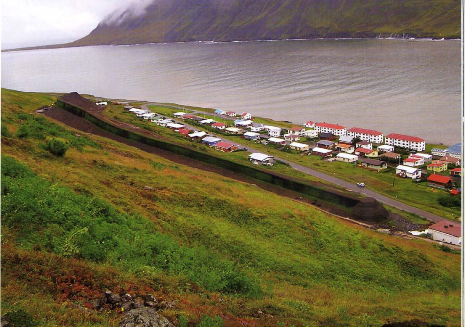
| An earth-retention system is now in place as an avalanche protector near the municipality of Siglufjörður in northern Iceland. The town rests at the base of steep mountainsides that are covered with snow for much of the year. Five barrier systems, each more than 1 mile long and 15-20ft high, were used to create the avalanche protection barriers.
