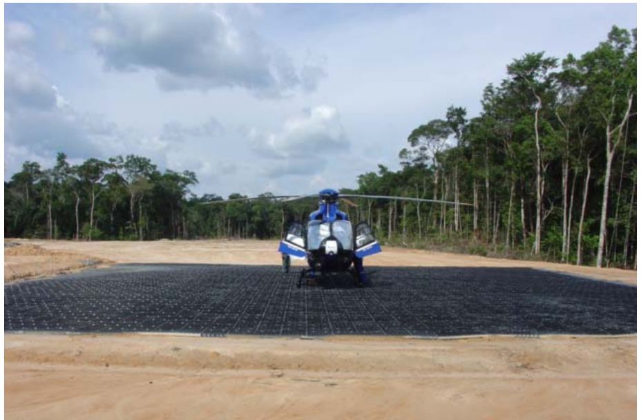
For areas where larger equipment and materials are dropped, a 20 m x 20 m area may be more typical. The material for this size helipad could be transported in 32 sub-assemblies and easily assembled by a two person crew in three days.
