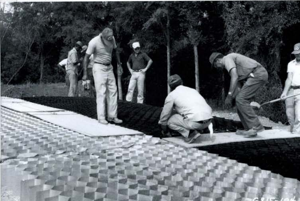
| Side-by-side cost/performance testing of a geocell (termed “roadbase”) and aluminum geocells at the Waterways Experiment Station in Vicksburg, Miss., circa 1979.
