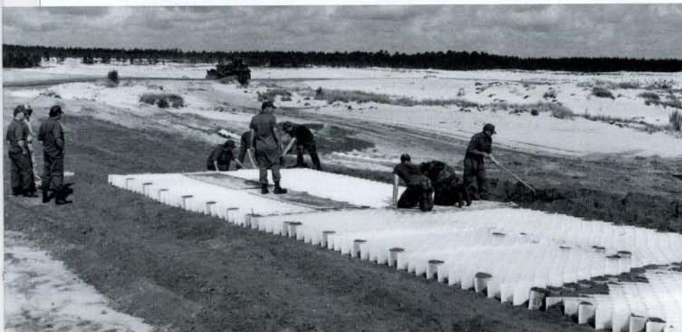
| U.S. Army Corps of Engineers testing a nonpigmented, non-UV-stabilized polyethylene grid confinement system at Camp Blanding, Fla., in the early 1980s.
