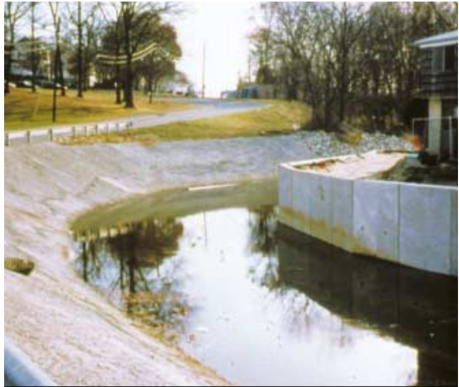
Photo 2: Concrete infilling of the geocell sections on the 1v:2h channel side slopes.
