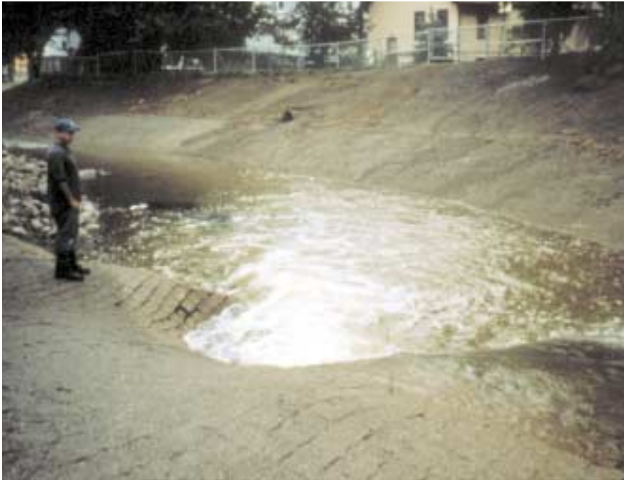
Photo 4: Geocell-protected section of the channel suffered minimal damage from Hurricane Floyd.
