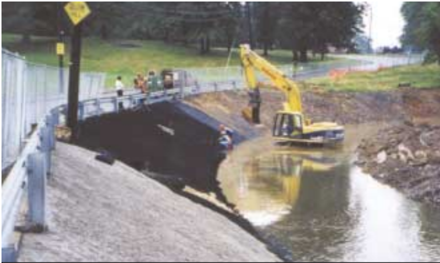
Photo 1: Geocell sections underlain with a geotextile are placed on the prepared segment of the channel bend.
