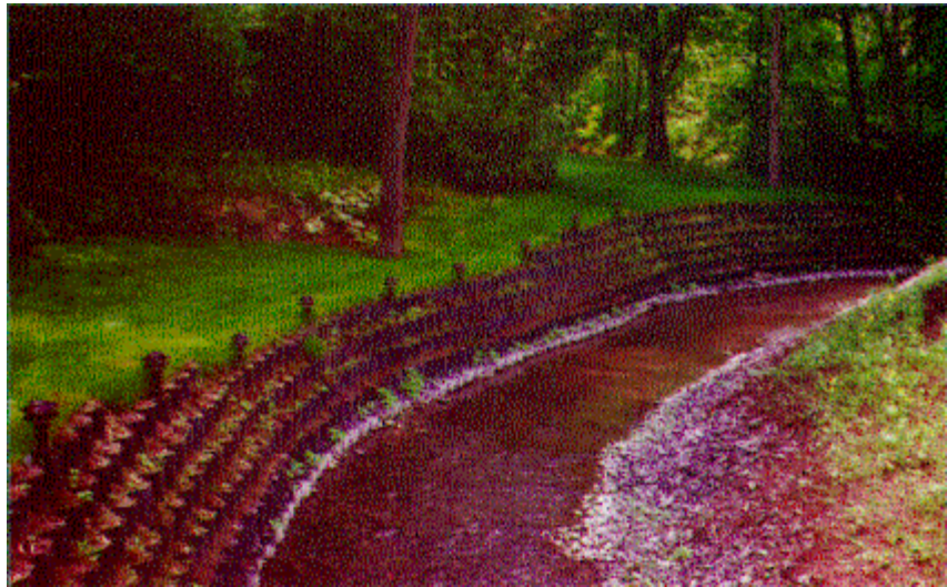
The balance of the channel lining system consisted of 200 mm deep, textured and tendoned Geoweb sections.
