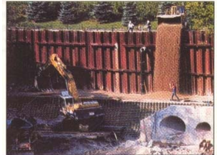
Top: The first layers of the 150-ft wide geocell-faced reinforced earth embankment are constructed to cover an aging sheet pile system.
