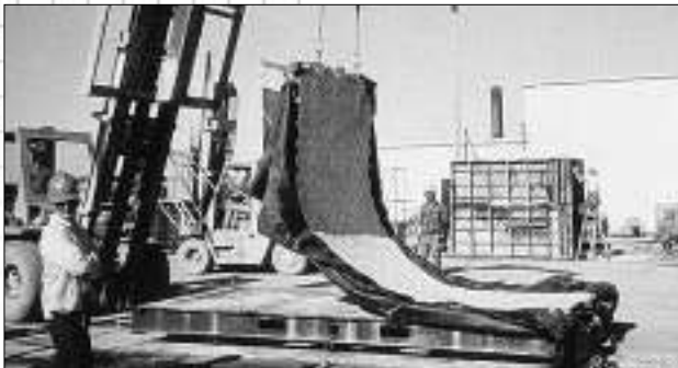
An installation with concrete-infill provides a more durable boat ramp to support heavier boat requirements and help prevent shoreline scouring. The GEOWEB sections were filled with concrete offsite and the cured concrete "mat" transported to the site.
