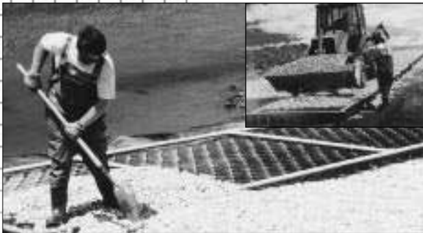
Gravel infill is distributed into sections with a front end loader. Hand tools may be used to aid in spreading the fill into the cells.
