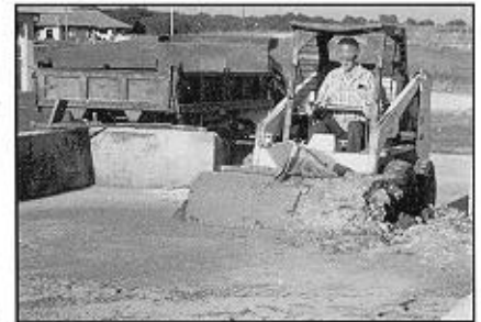
3. The confined filtration sand easily supports the loader used to remove dried sludge.
