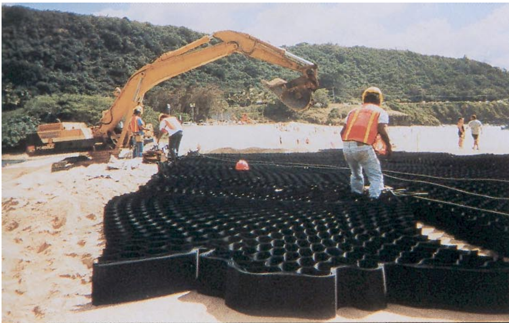
Material sections 8 ft by 20 ft are placed three across to create the 24-ft wide, 1,000-ft long roadway.
