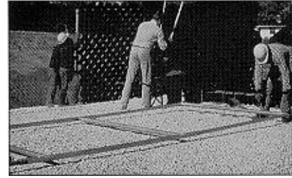
The polyethylene geosynthetic material is installed in 1984. Aluminum stretcher frames, used to expand the material, are removed after the material is infilled.
