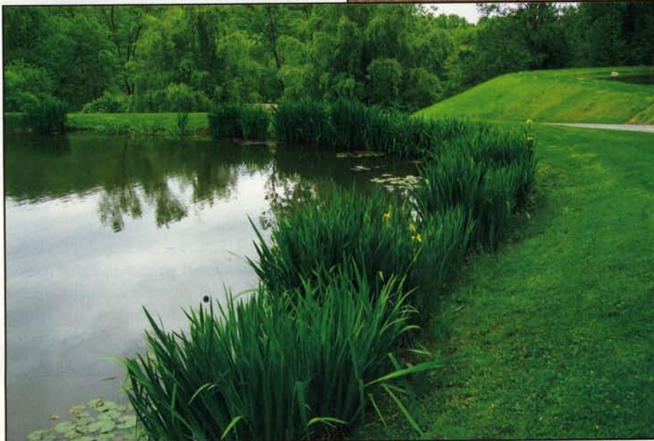
Topsoil within the geocell sections creates a planting medium for the desired water plants.
