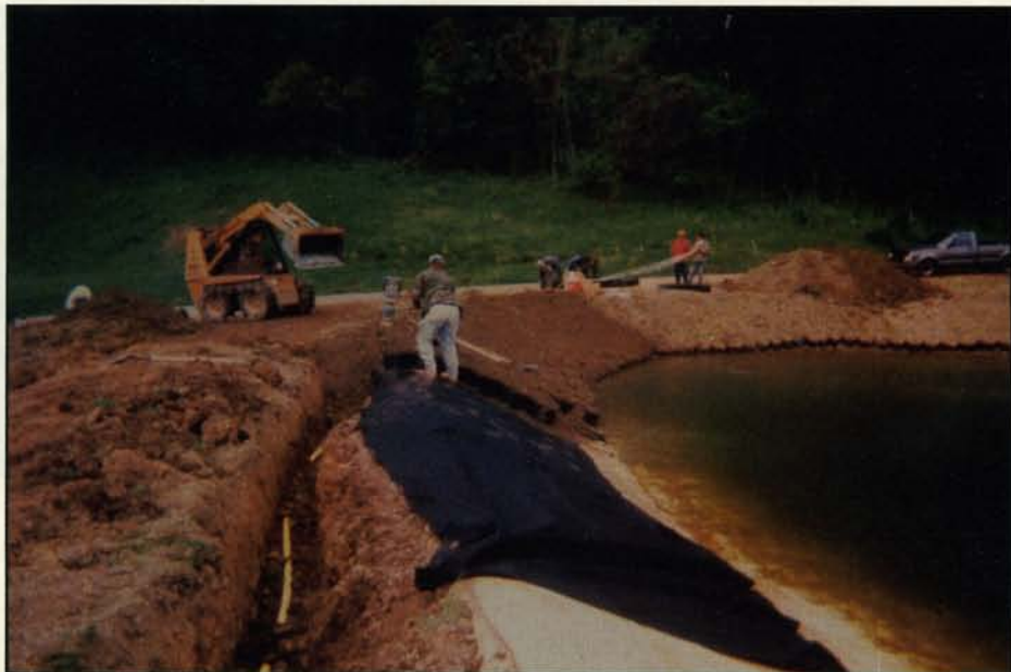
Geoweb sections are secured over the geotextile and geomembrane layers with tendons tied to a deadman anchor.
