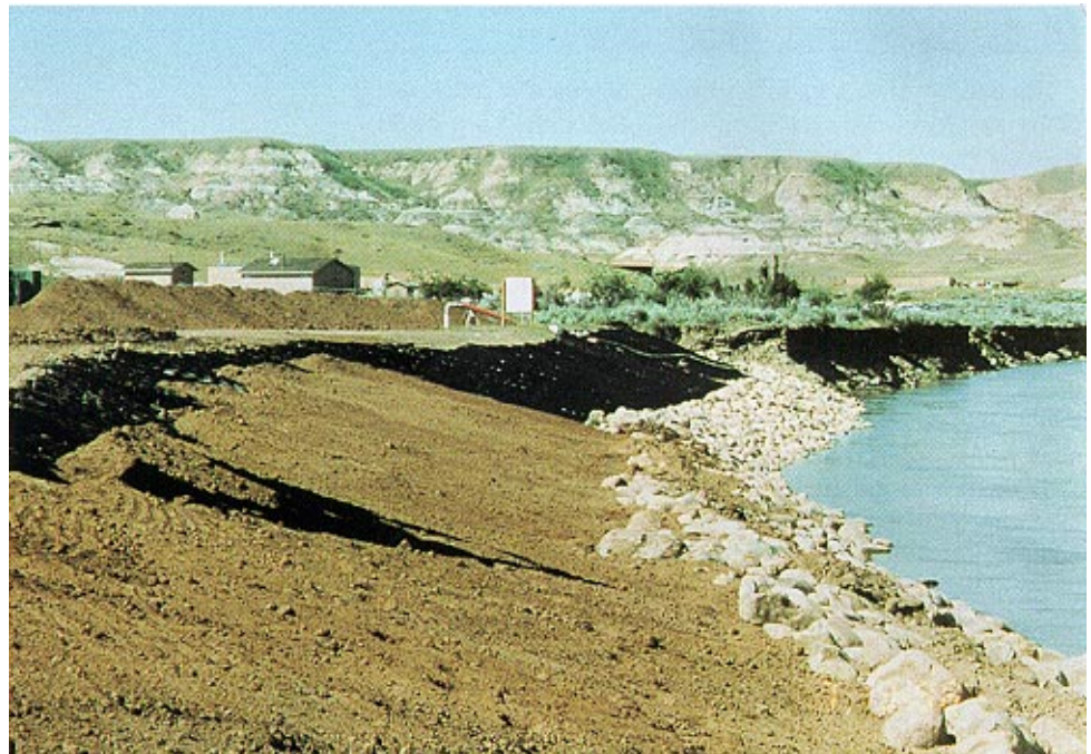
After installation, the geocells were filled with topsoil and seeded with a native grass mixture. The geocells increase the vegetation's natural resistance to erosive forces and protect the root zone from soil loss.
