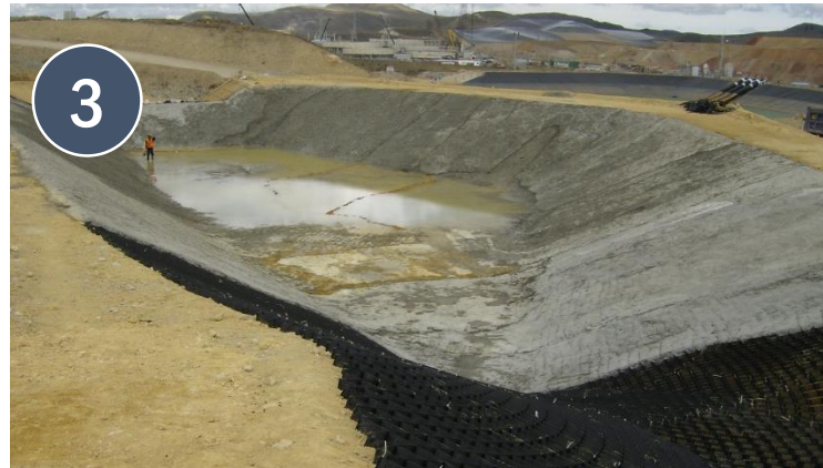
Basin Containment (p. 19-20)
